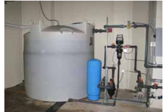
Amiad and UV Rainwater ReUse System
